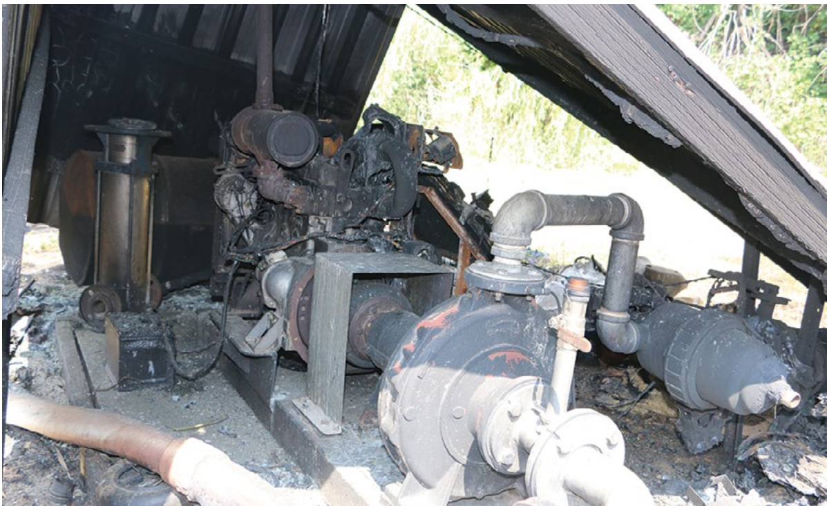
Figure 21. Damage to irrigation pumps delays efforts to re-establish irrigation in the orchard after the fires.
