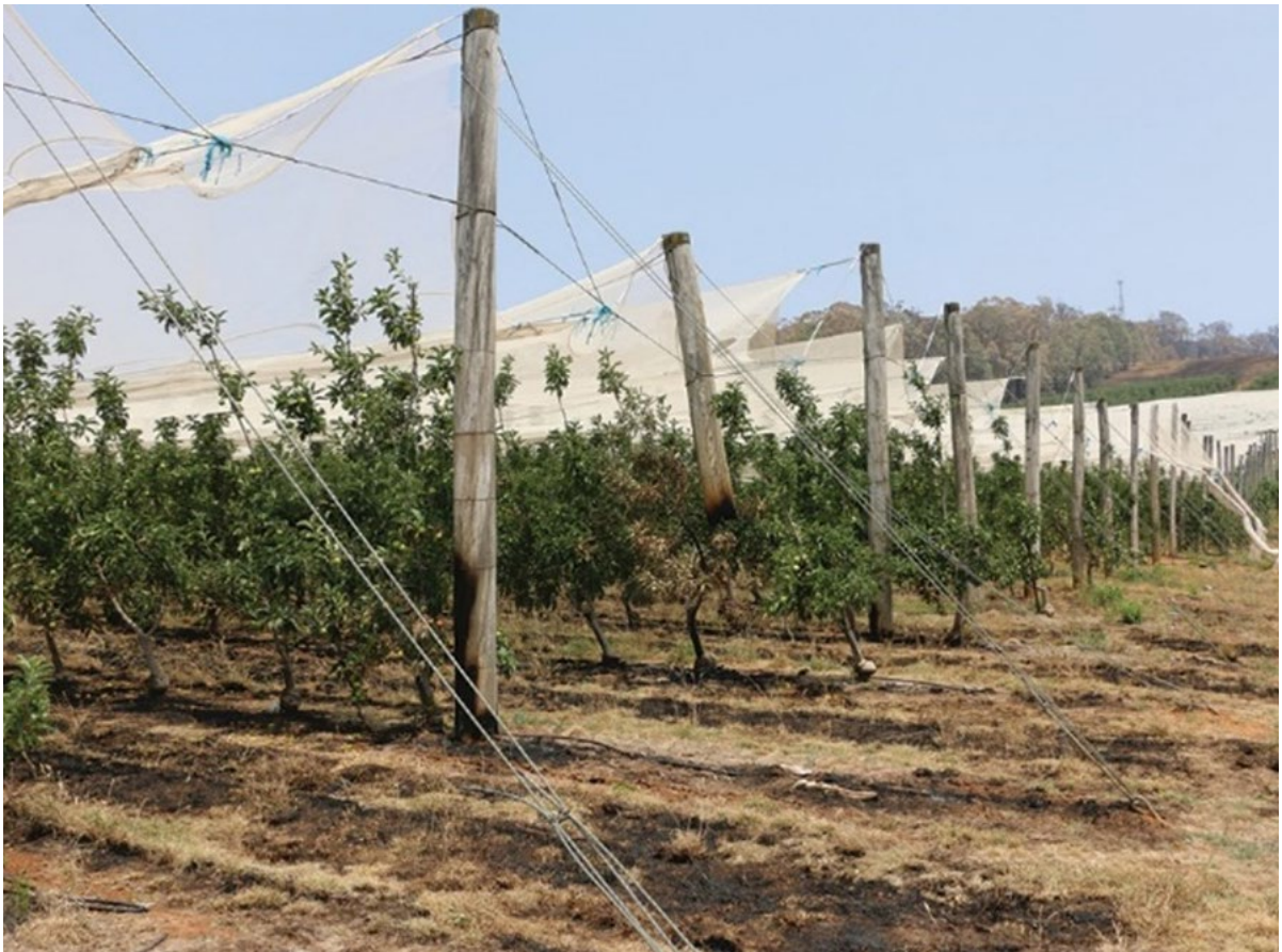
Figure 19. Structural damage to timber strainer posts in a block with structured hail netting.
