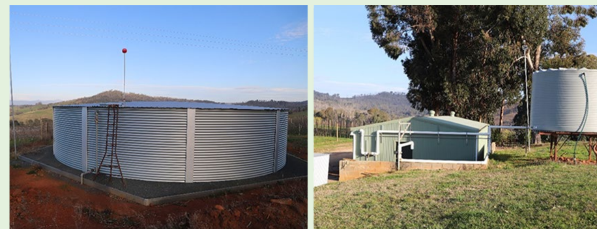
Figure 50. Water supplies should be secure, uninterrupted and offer high flow for fast filling of firefighting units. Ardrossan Orchards installed high capacity, fire resistant steel tanks, gravity feed and large diameter pipes to facilitate fast filling.
