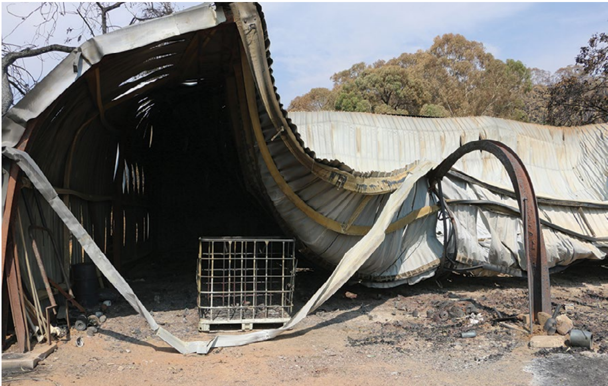
Figure 20. Harvest bin storage sheds can generate enough heat to soften and bend steel beams.
